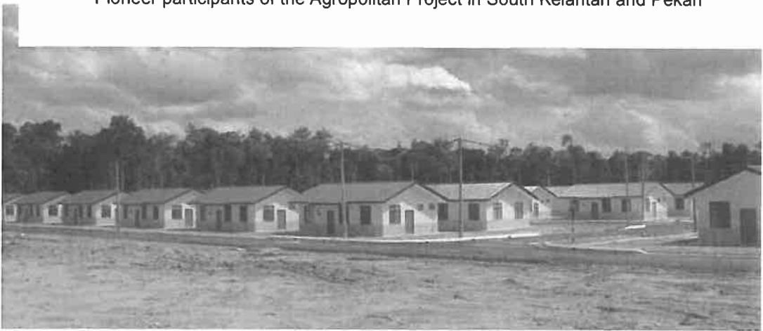
The construction of new houses for participants implemented in stages in Pekan
