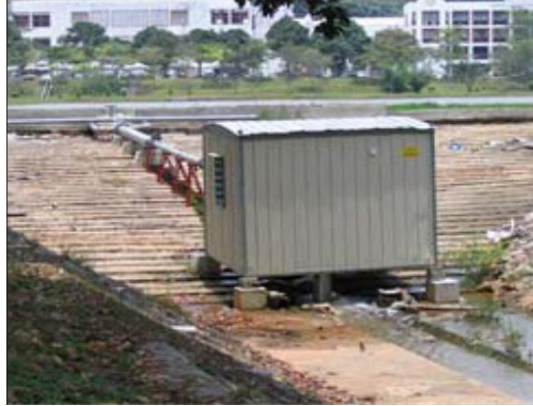
Figure 4. Pico Hydro Generation in UKM
