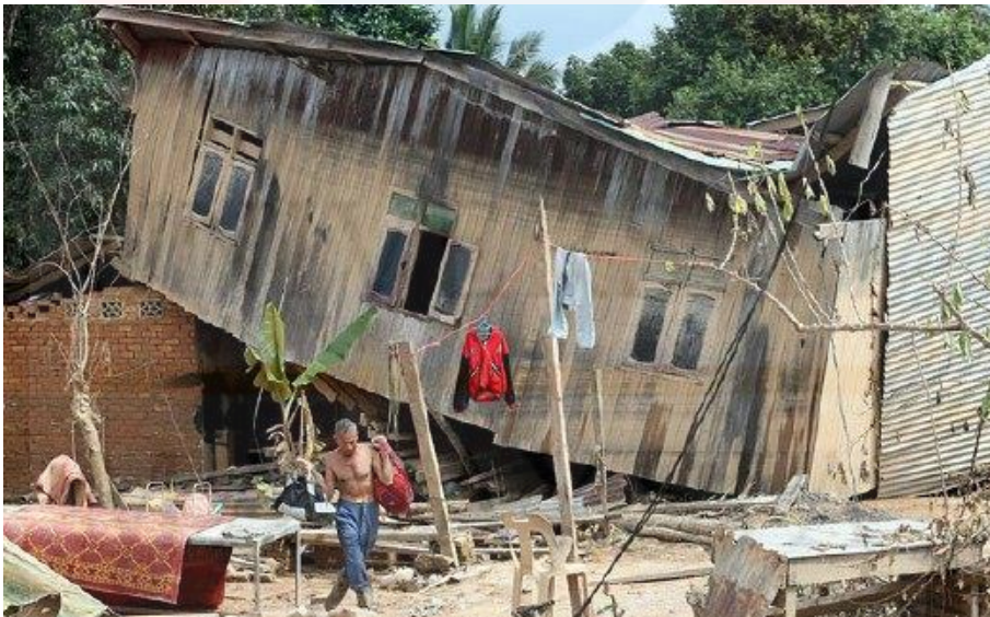
Figure 2.2: Impact of flood in Kuala Krai (Source: Berita Harian, 2014)
