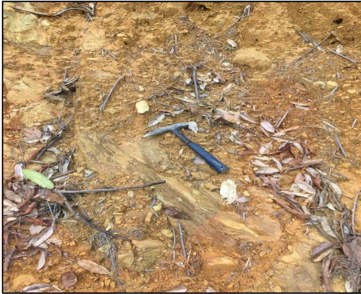
Figure 5.5: Bedding structure at the slope failure.
