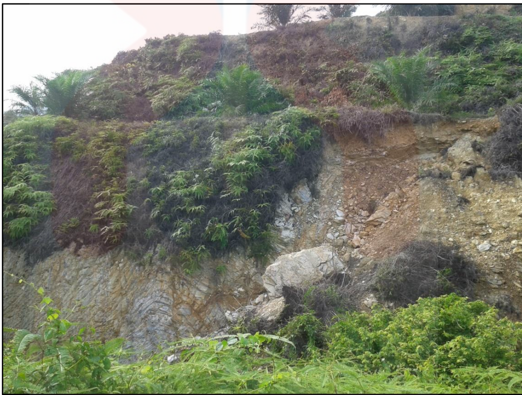
Figure 5.2: Overview of slope where slope failure 1 occurred.
