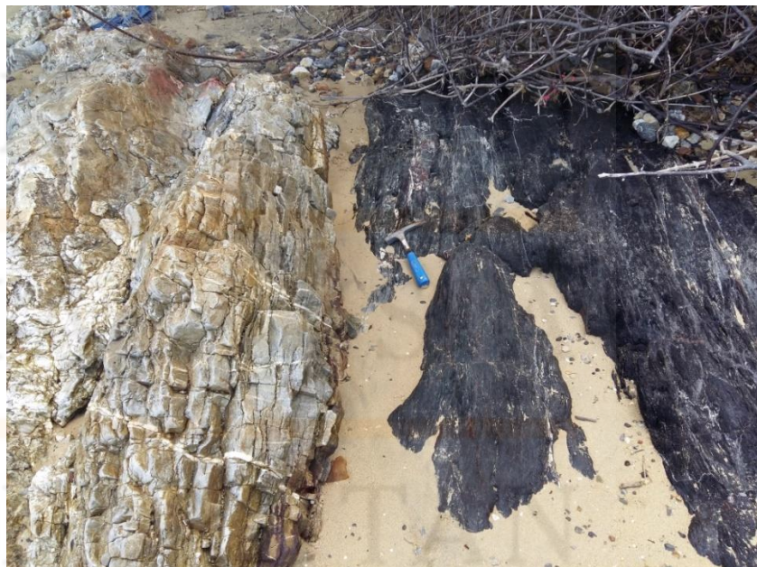
Figure 4.41: The joint are more likely to develop in sandstone body compared to shales body.
