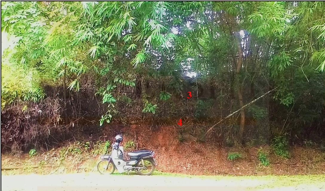
Figure 5.3 Slope failure at location 2
