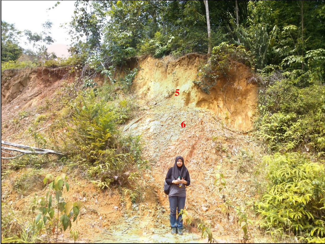
Figure 5.4 Slope failure at location 3
