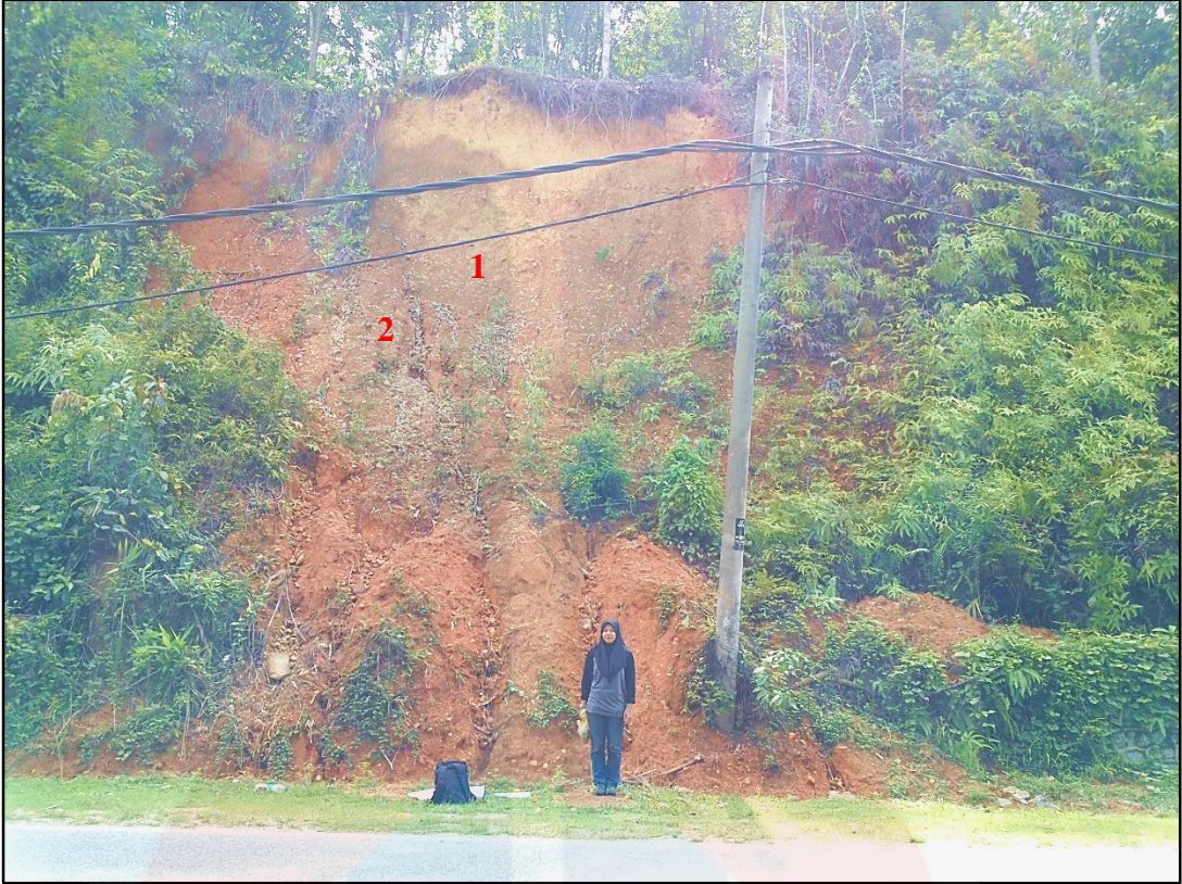
Figure 5.2 Slope failure at location 1
