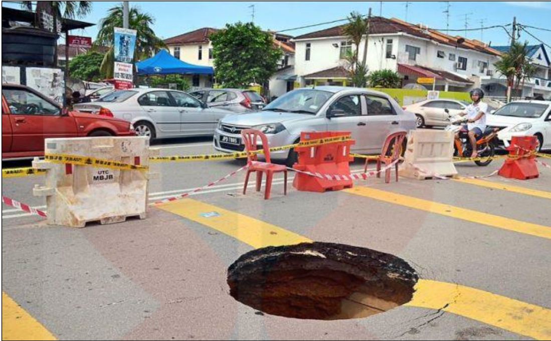
Figure 1.1: Sinkhole along Jalan Kempas, Taman Megah Ria in Johor Bharu.
