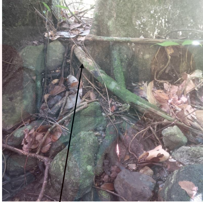
Figure 4.2: Root wedging breaks along the joints.
