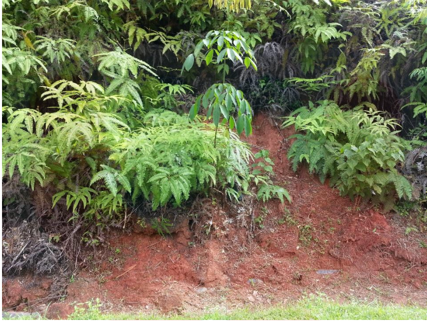
Photo E5: Slope failure 5
