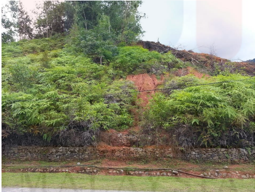
Photo E4: Slope failure 4 (Coordinate: N 05° 24' 33.1", E 101° 56' 07.3")
