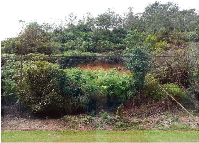
Photo E7: Slope failure 7
