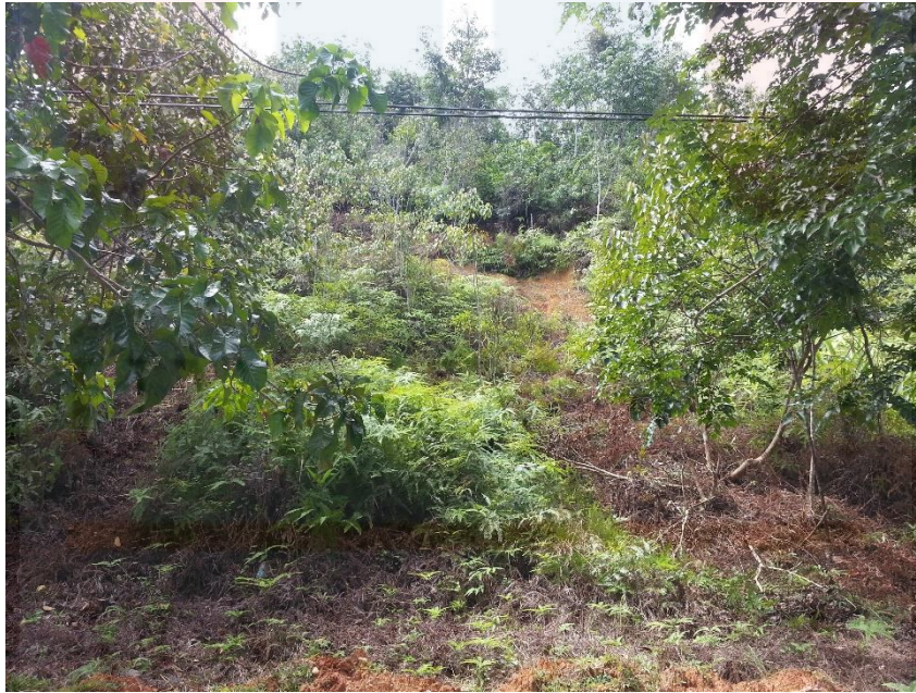
Photo E8: Slope failure 8
