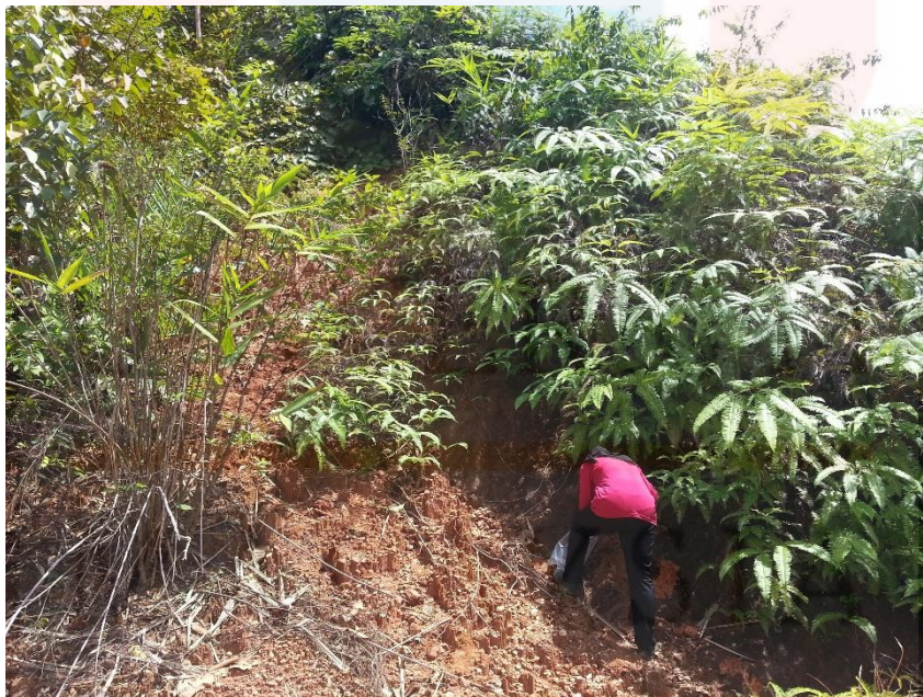
Photo E2: Exposed part of slope failure 1 (Coordinate: N 05° 24' 44.0", E 101° 55' 54.2")
