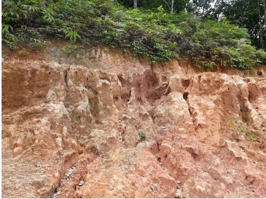
Figure 4.15: Gully erosion at 05^{\circ}24'51.0'' , 101^{\circ}55'49.0'' .
