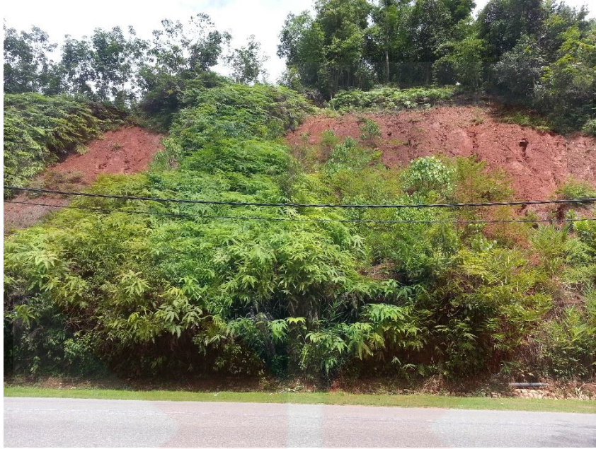
Photo E3: Slope failure 2 and 3 (Coordinate: N 05° 24' 41.9", E 101° 55' 55.1")
