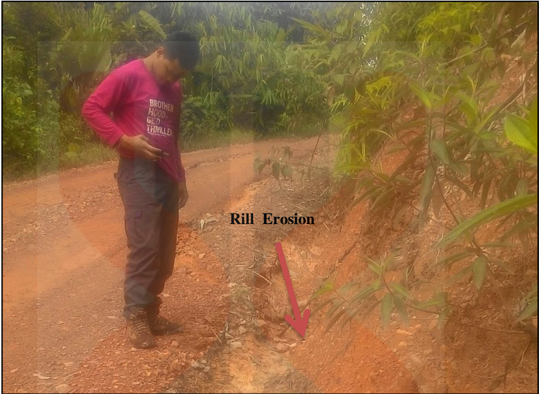
Figure 4.12 : Rill erosion can be seen clearly (red arrow)
