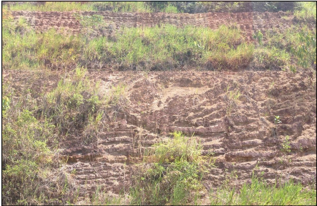
Figure 4.11 : Biological weathering on sandstone outcrop, the root from the vegetation make crack on the outcrop.
