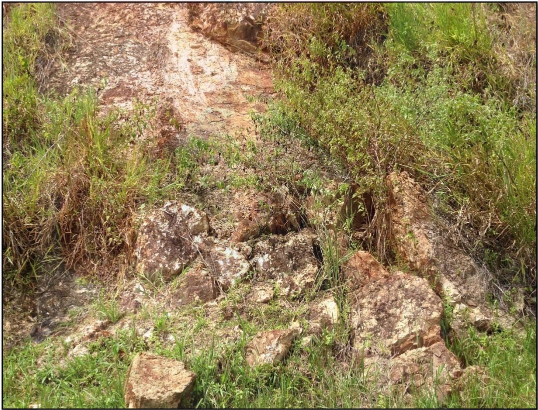
Figure 4.14 : The occurrence of rock fall on the sandstone outcrop besides the main road in study area.
