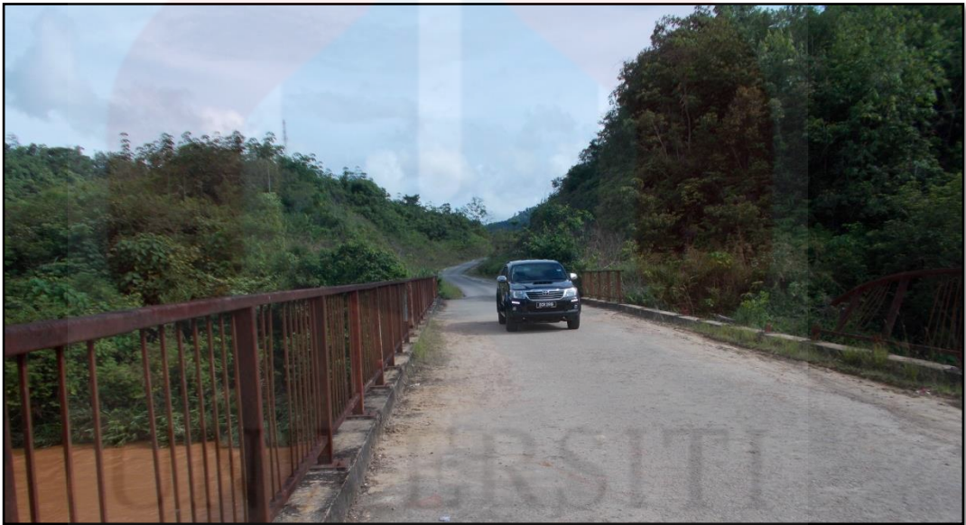
Figure 1.11 : The bridge at Sg. Berok connecting Pos Blau with Gua Musang-Cameron Highway.
