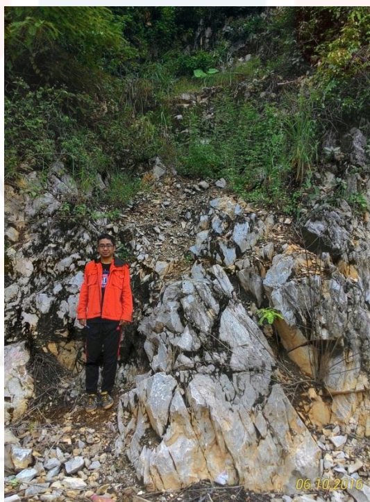
Figure 4.13 : Rock fall near the main road to Kampung Batu Papan
