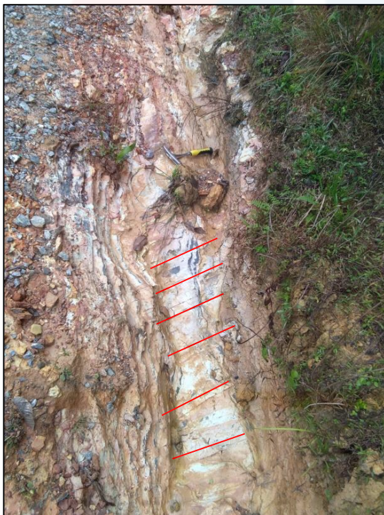
Figure 4.62: Parallel joint on phyllite outcrop in palm vegetation area. The picture was taken at station 19.
