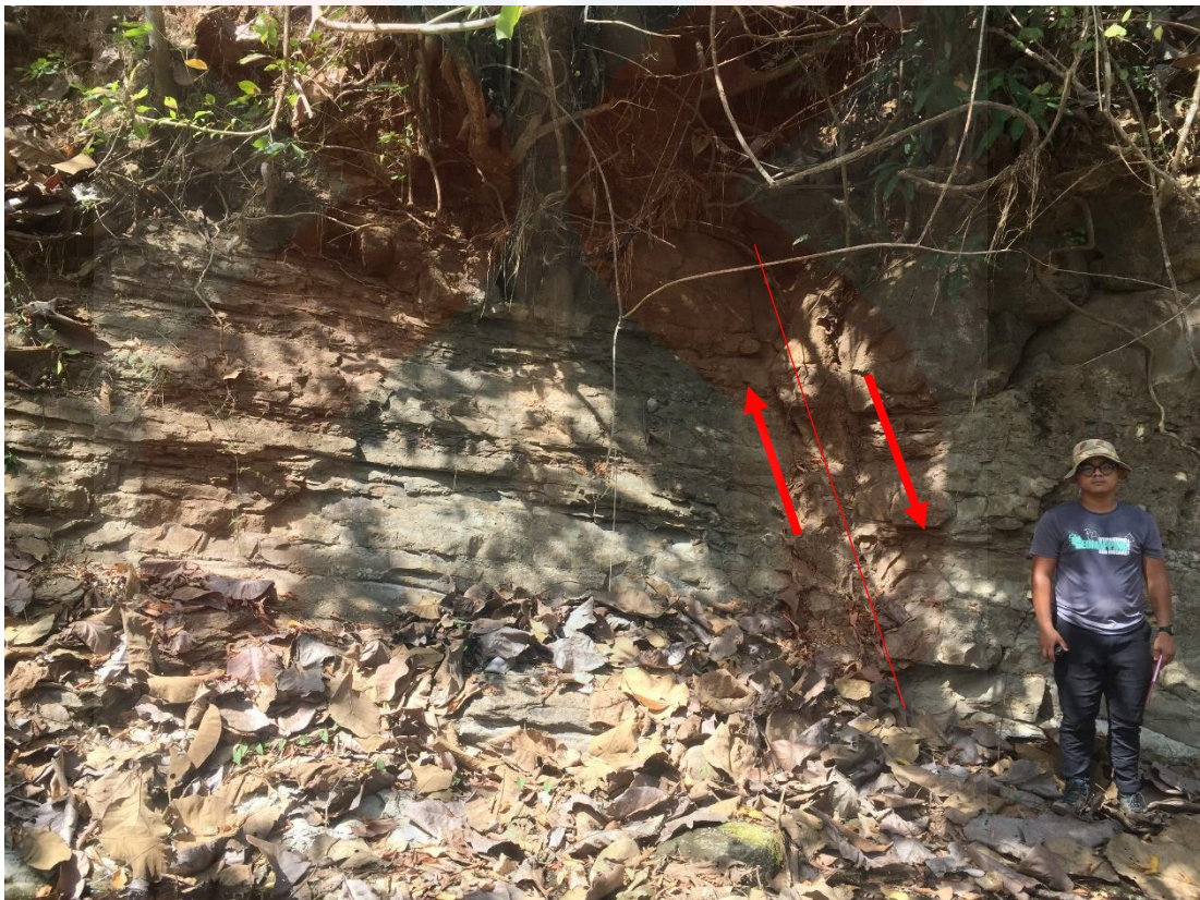
Figure 4.14 Show the direction normal fault (red arrows) and its fault plane (Red line)
