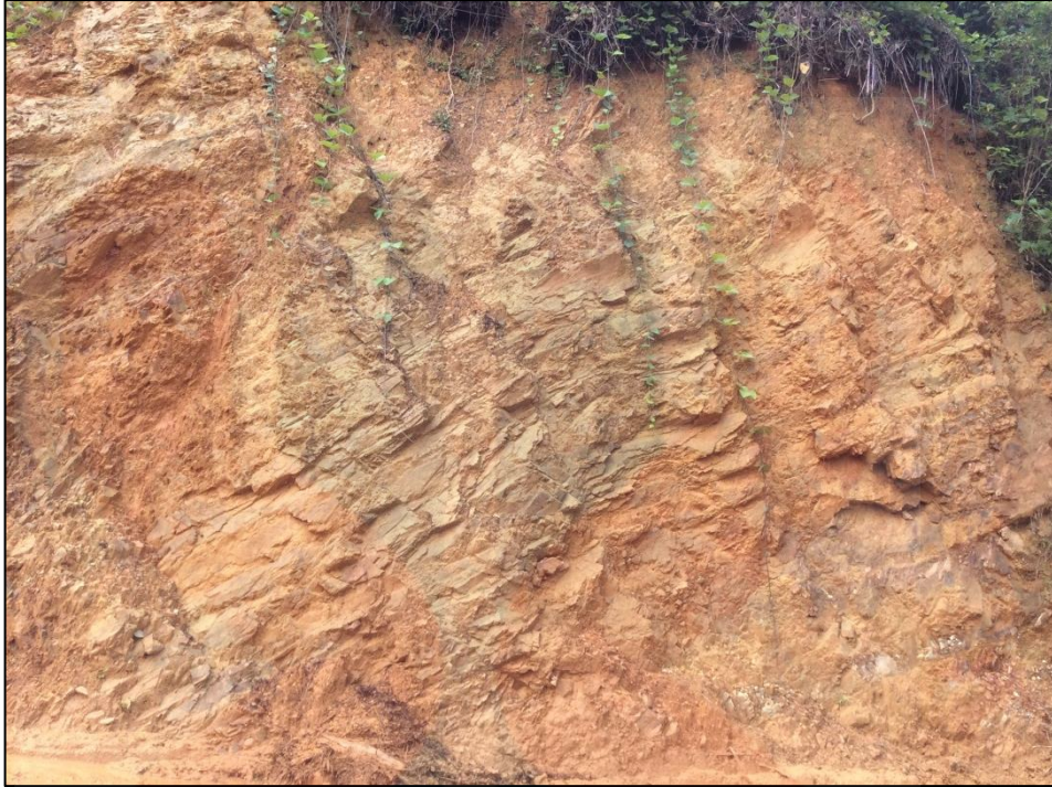
Figure 4.32 Shear joints at slate rock
