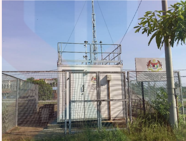
Figure B2: Monitoring station of Department of Environment in Kemaman
