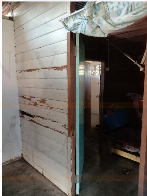
The signs of the presence of termites
