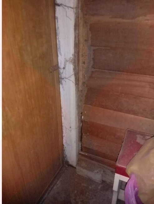
Wooden walls worn out by termites
