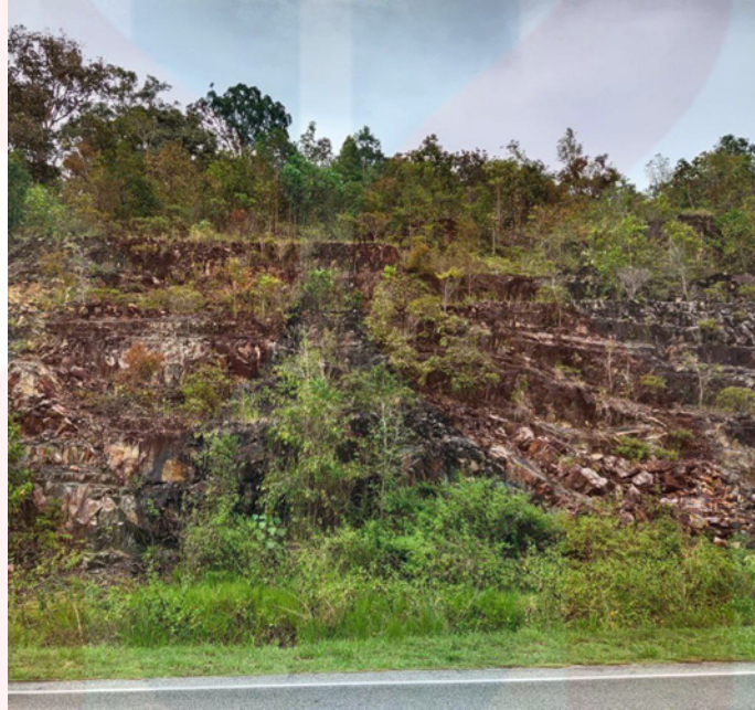
Figure 4. 17: The Fault at the study area
