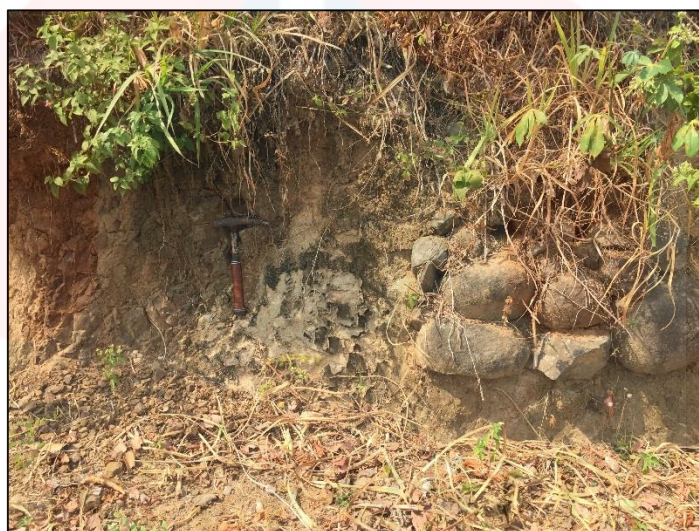
Figure 4.2.6: Biological weathering by a tree
