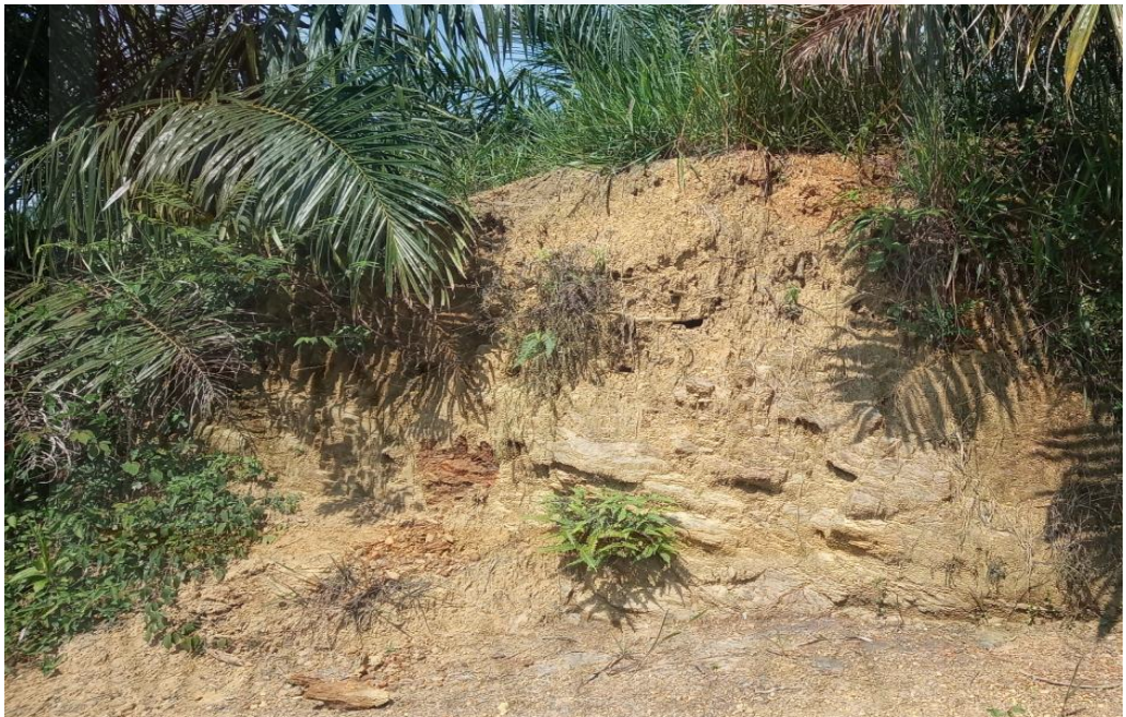
Figure 4.9: Example of biological weathering
