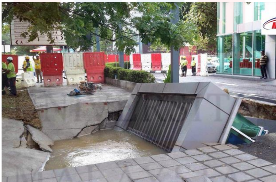
Figure 1.1: Sinkhole That Occurred at Bukit Bintang
