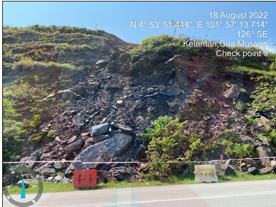
Figure 5. 3: Landslide occurred along the major road at checkpoint 9. The size of failure is massive
