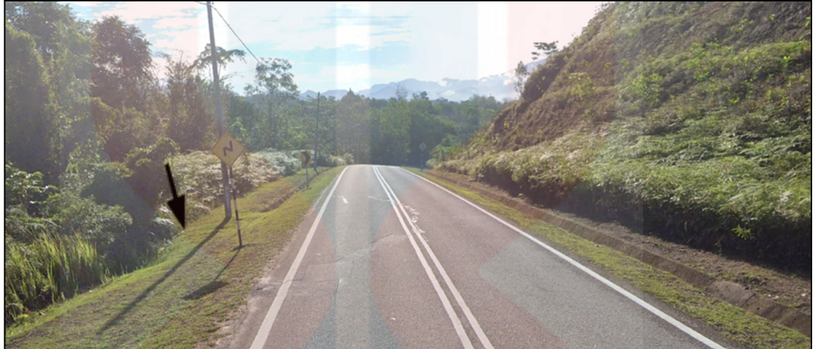
Figure 5. 2: The tension crack on the Gua Musang road, which shown the sign of slope movement.
