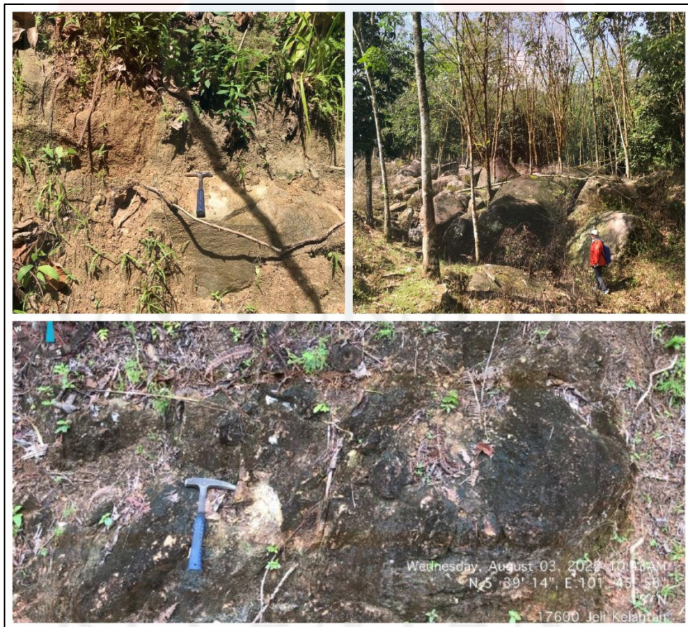
Figure 4.12: Biological weathering in the study area causes by tree, root plants, and black algae.
