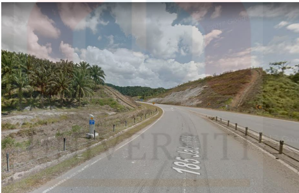
Figure 5.3: shows the steep slope at the research area, Aring 5, Gua Musang Kelantan. (source: Google map, 2020)
