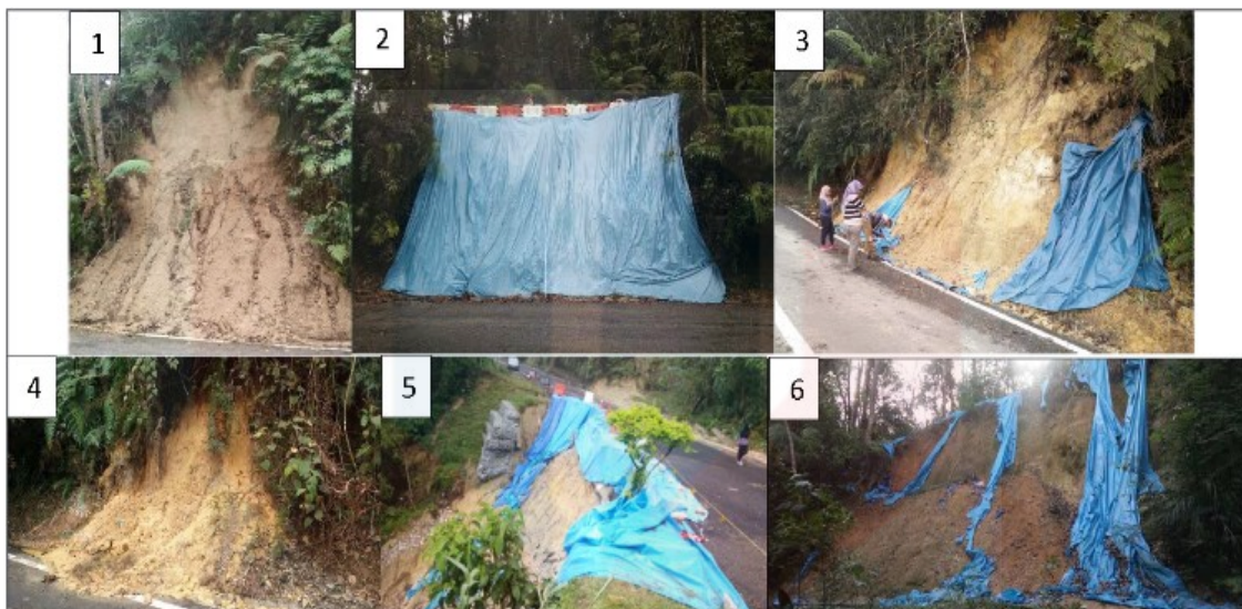
Figure 5.5 Landslide Hazard at Fraser Hill
